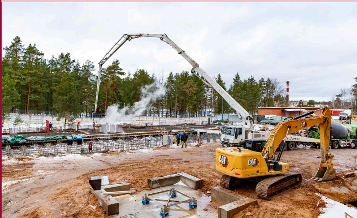
21 December. Pouring the first cubic meters of concrete into the foundation of the U-400R experimental building
